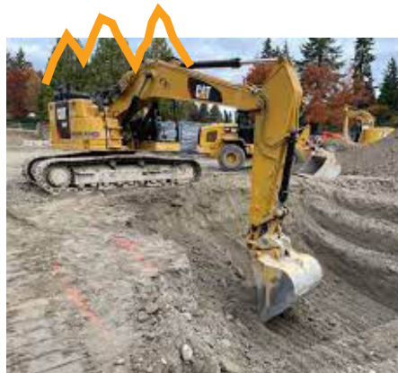
Construction activity with three western redcedars outlined in the background. Photo from November 2021.
